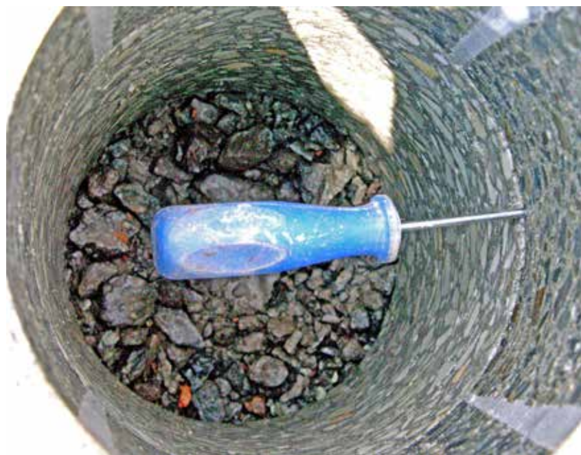
Fig. 10: Absent bond between paving block and foundation concrete
